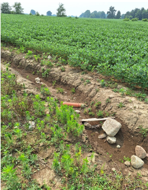
Soil erosion and exposed tile in Union County prior to grassed waterway installation
